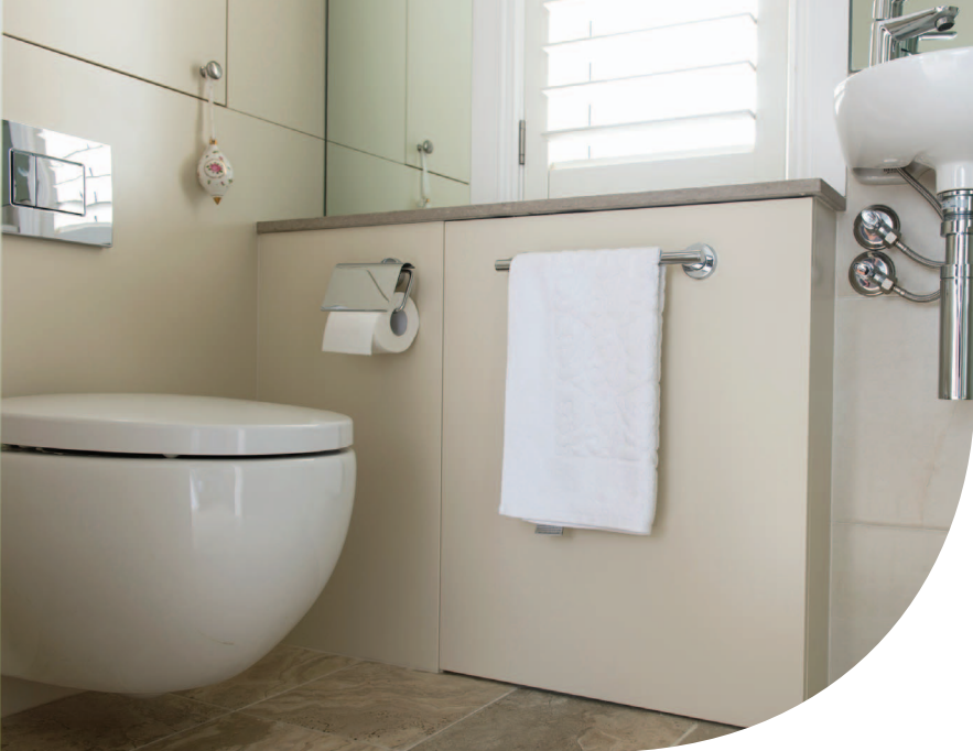
The Sanipack was used to install an ensuite off the main bedroom and a powder room next to the main living area.
